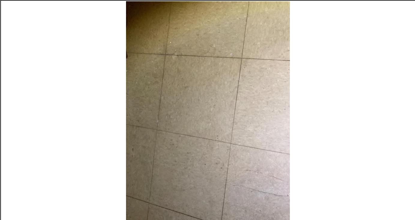
Photograph #5 Positive ACM located in 9"x9" vinyl floor tile located in building 18, rooms 35 and 45.
