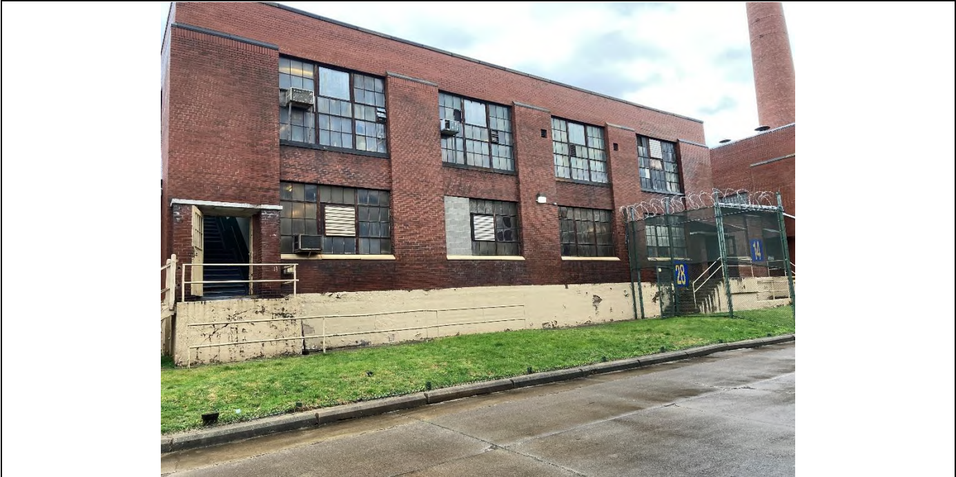
Photograph #1 SCIP Building 28 – Maintenance Shops. No ACM was detected in this building.
