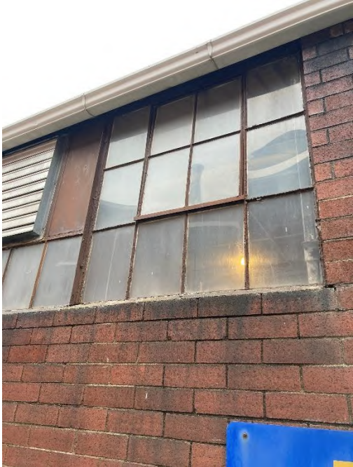
Photograph #2 | Positive ACM located in exterior window caulk located in building 10
