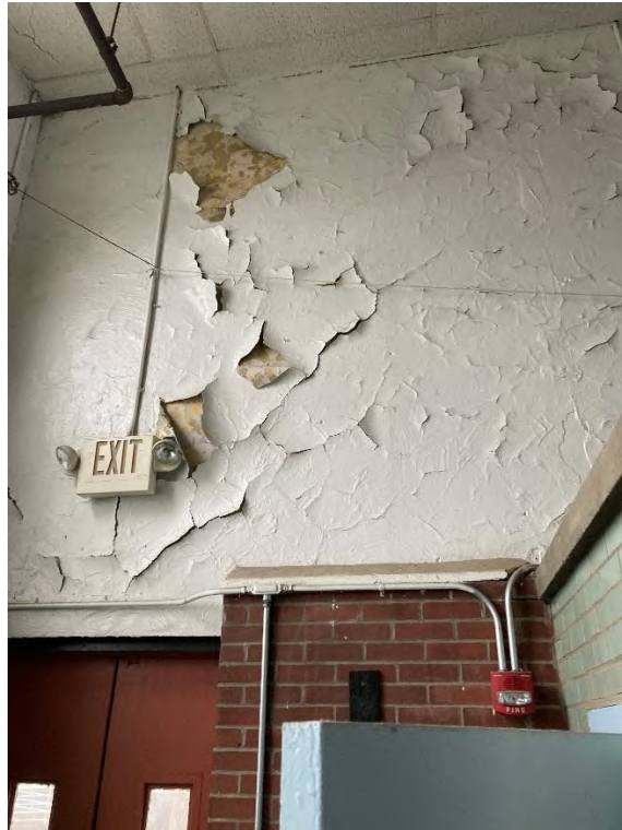
Photograph #2 | Positive ACM located in wall and ceiling plaster located in building 8
