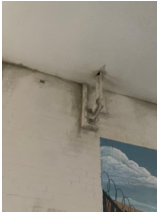
Photograph #2 | Positive ACM located in thermal pipe insulation located in building 16, rooms 1, 3, and 5.
