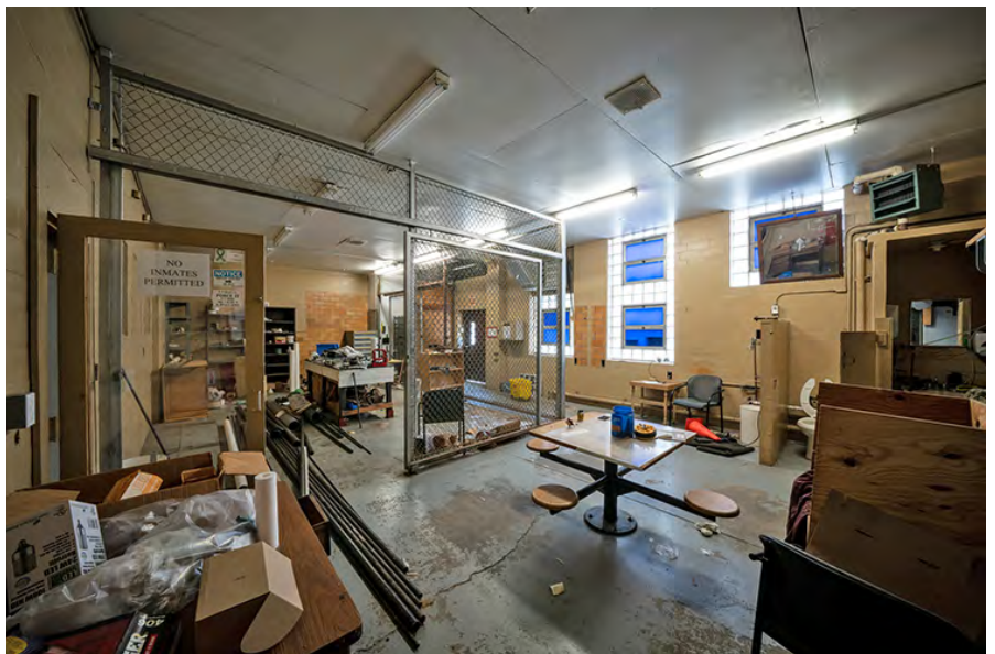
Photo 62. Maintenance Building interior, looking northeast, showing the Plumbing Shop.
