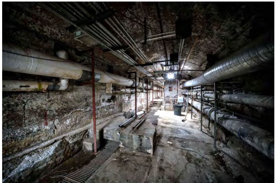
Photo 26. Main Penitentiary Building interior, basement under Housing Unit D, looking north, showing the distribution of mechanical, electrical and plumbing services, stone walls and floor, and arched brick ceiling
