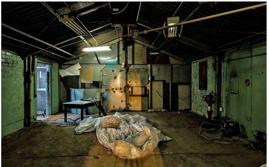
Photo 51. Correctional Industries Shop Building interior, infill connector between the Tag and Metal Shops, looking west. The electrical substation is beyond the end wall.
