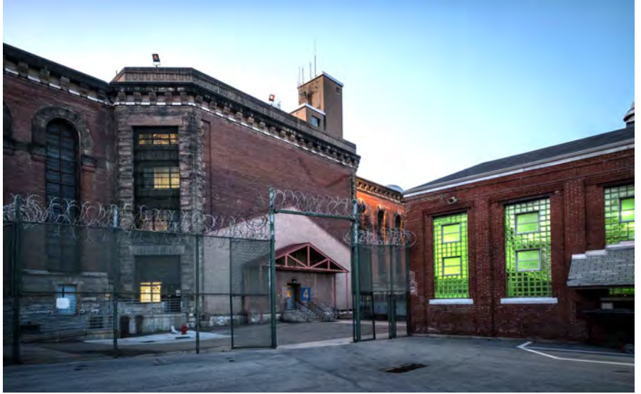
Photo 15. Main Penitentiary Building, east facade, looking northwest from the Main Yard, showing the Rotunda (center) and Auditorium (8) to the right.
