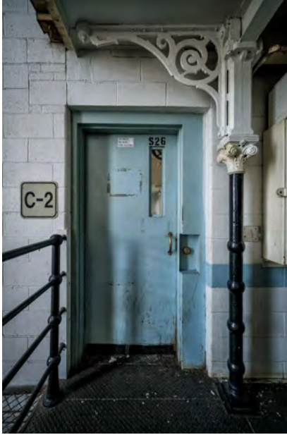
Figure 123. Photograph showing some of the structural and ornamental cast iron found throughout the Main Penitentiary building. The Female Ward had similar cast iron brackets (Matthew Christopher).
