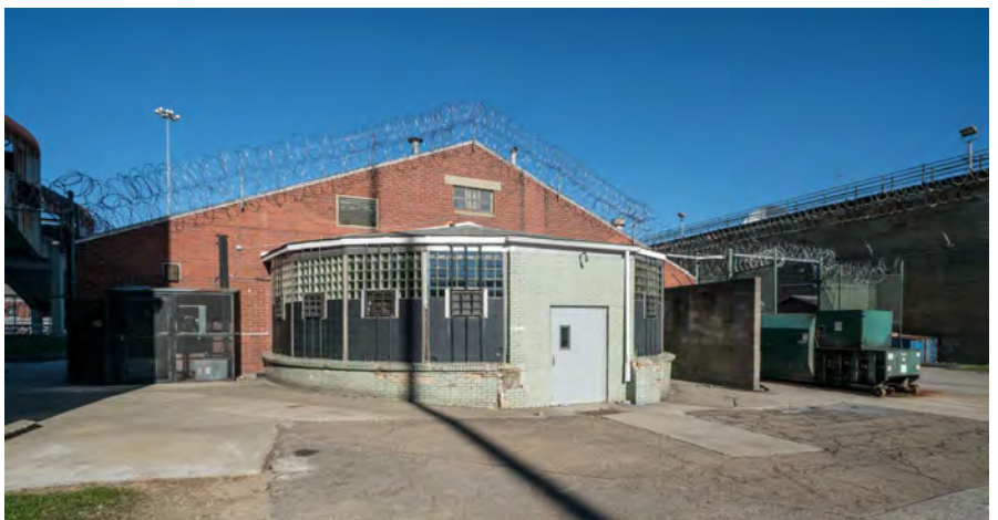
Photo 54. Dining Hall, south facade, looking northeast, showing the red brick south wall of the 1957 addition and the half-round dish washing room in mint green glazed brick and glass block.
