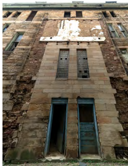
Photo 8. Warden's Residence, rear facade, looking west, showing where the porte cochere and bridge once existed.
